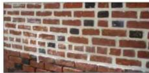
Example of mismatched mortar
